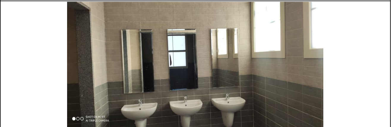
Supplying water taps with water conservation units (Alexandria University, Egypt)
