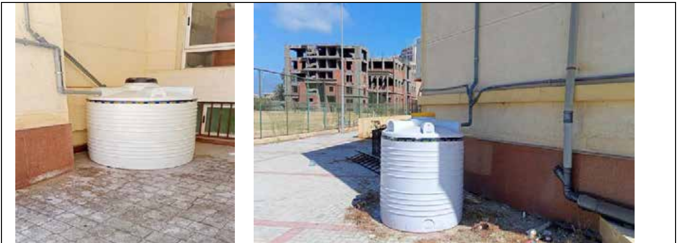
Air conditioning water collection and reuse unit - Faculty of Engineering
