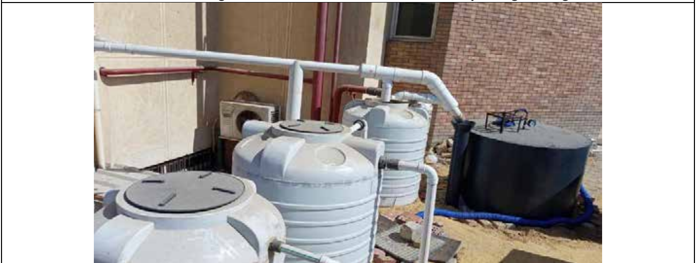
Wastewater treatment unit at the Faculty of Engineering
