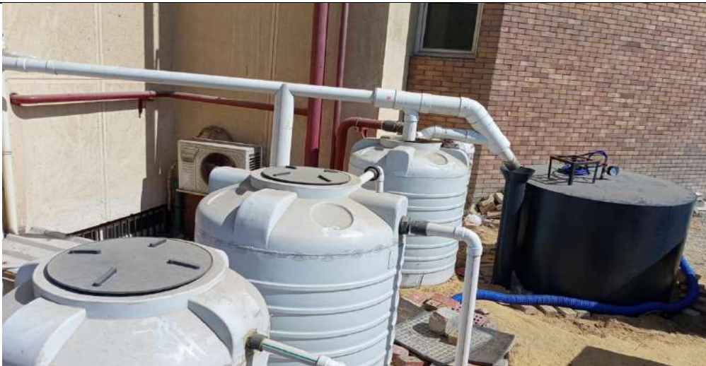
Wastewater treatment unit at the Faculty of Engineering
