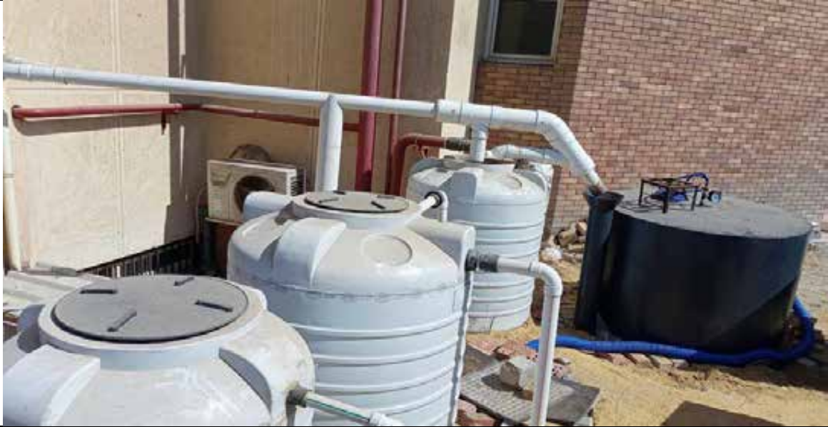
Wastewater treatment unit at Faculty of Engineering
