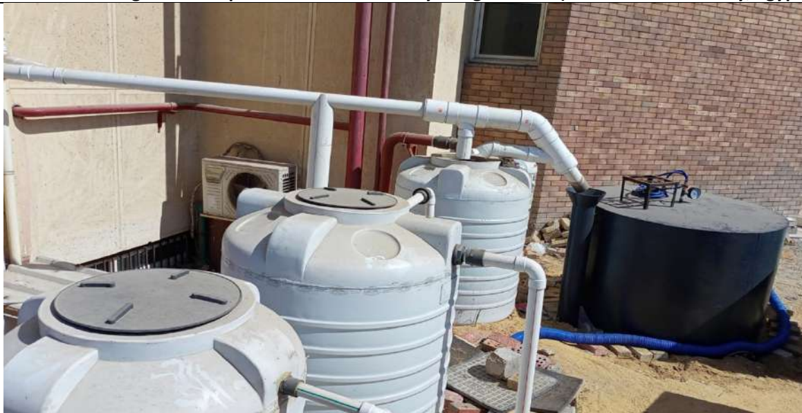
Wastewater treatment unit at Faculty of Engineering
