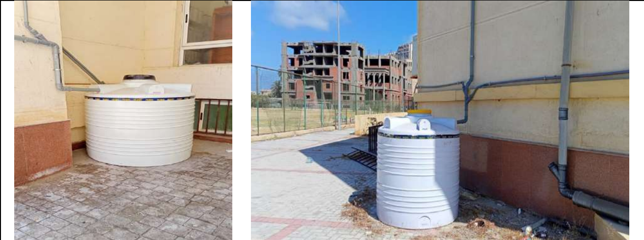
Air conditioning water collection and reuse unit - Faculty of Engineering
