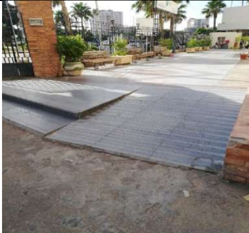
Replacing steps with ramps for disabled people (Faculty of Pharmacy - Alexandria University)
