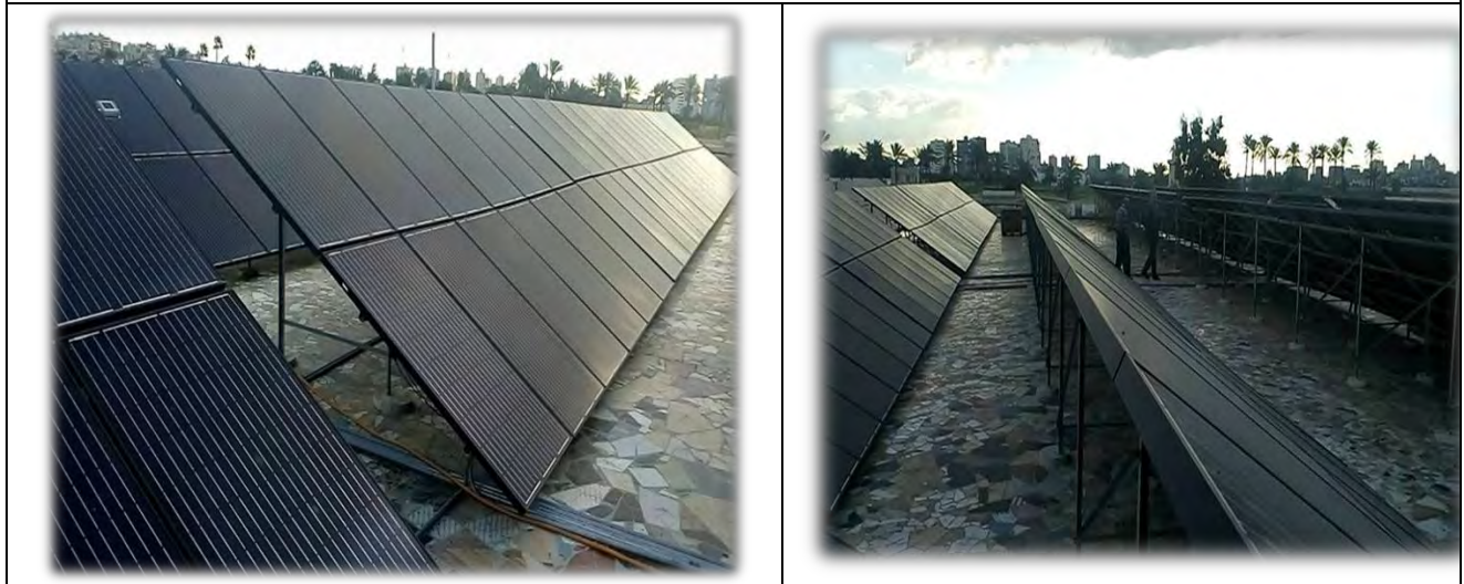
Solar Panels (Solar Energy Center at the Faculty of Agriculture - Alexandria University)
