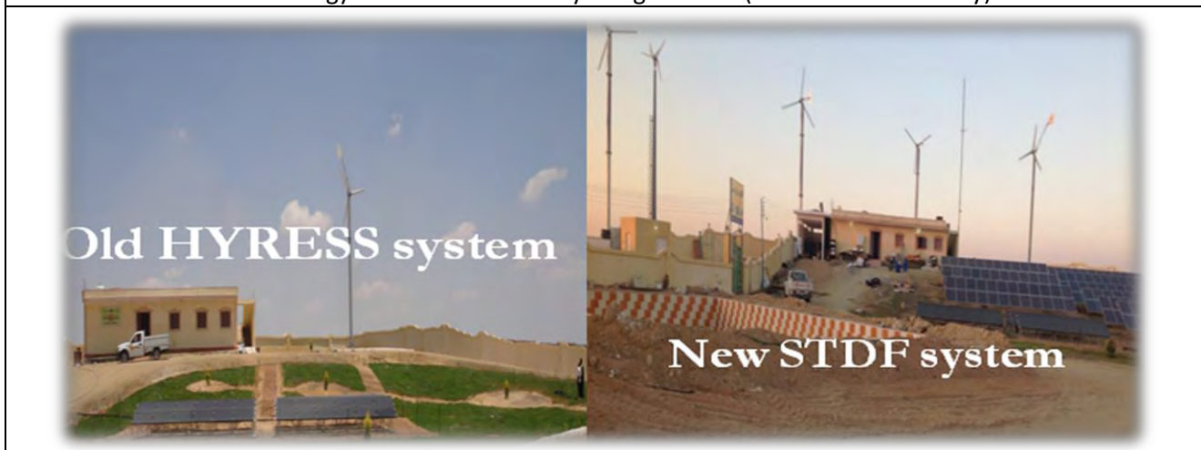
Windmill and Solar Panels (Solar Energy Center at the Faculty of Agriculture - Alexandria University)
