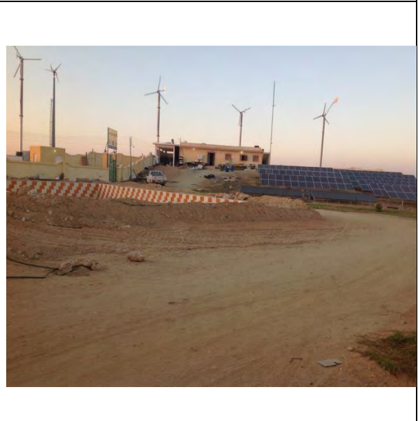
100 KW Hybrid Wind/PV System (50 KW PV and 50 KW Wind)
