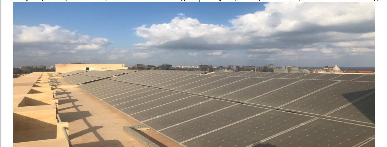
Solar photovoltaic with a capacity of 220 kilowatts on the 2000 m 2 roof top of the building of the Mechanical Engineering Department at the Faculty of Engineering
