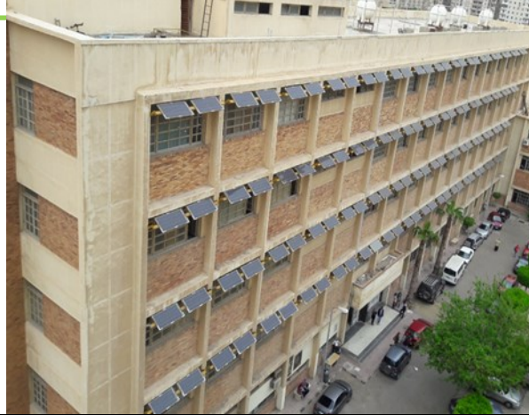
BIPV Façade Brise-Soleil System Solar Energy Project at the Faculty of Science (Alexandria University)
