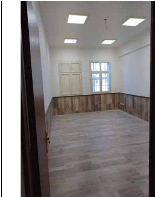
1. LED lighting and lamps (Abis Campus, Alexandria University)
