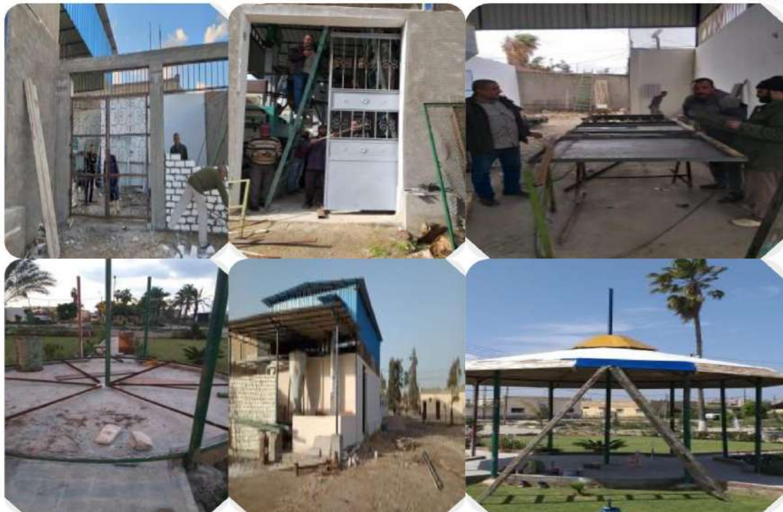
Recycling Program for both materials and equipment with metals and derivatives (Alexandria University, Egypt)
