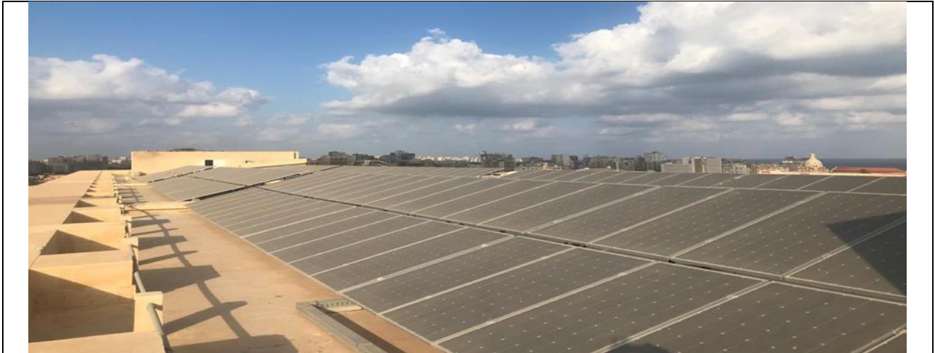
Solar photovoltaic with a capacity of 220 kilowatts on the 2000 m 2 roof top of the building of the Mechanical Engineering Department at the Faculty of Engineering
