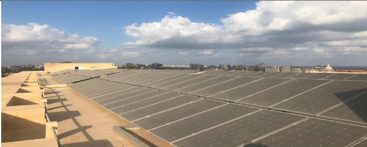
Solar photovoltaic with a capacity of 220 kilowatts on the 2000 m 2 roof top of the building of the Mechanical Engineering Department at the Faculty of Engineering
