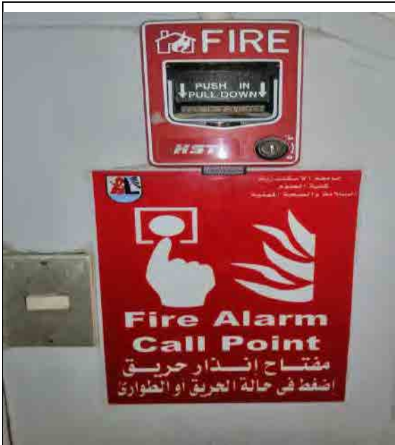
4. Fire alarm call point
